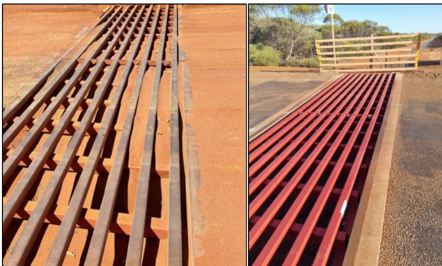
Before and after photos of the Karara Laneway Grid replacement by Karara Mining Ltd in the Shire of Perenjori.
